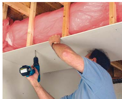
Skin the frame with drywall. Sheets of gypsum board add mass to the chased opening and deflect much of the airborne sound.
