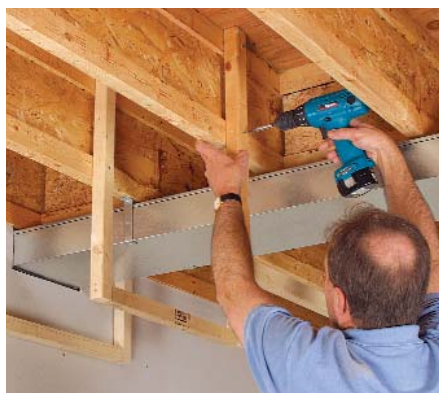
Cover the duct with a framed opening. Simple 2x3 frames assembled at the workbench are easily attached to floor joists with screws.
